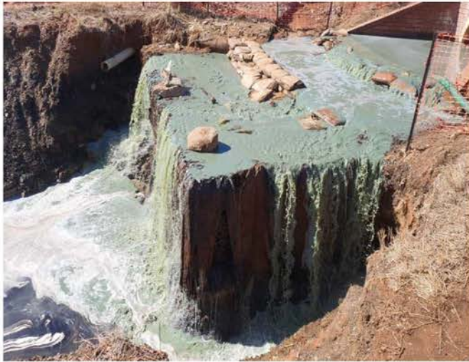
Highly contaminated water flowing from Outlet 1.
