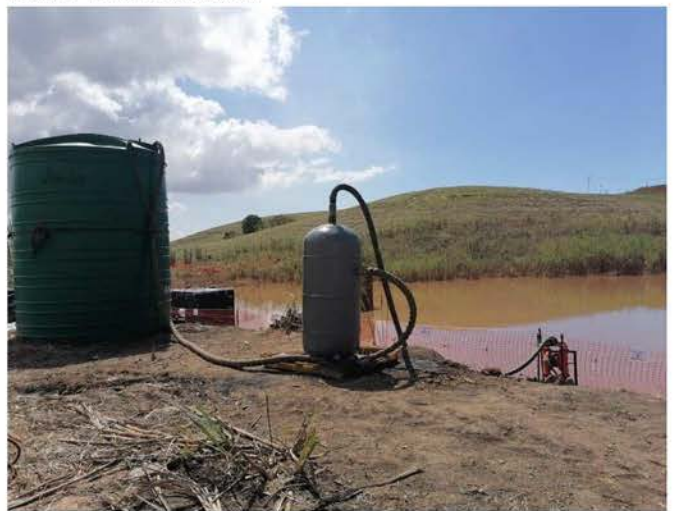
The team pumping contaminated water through the GAC pod into the JoJo tank.
