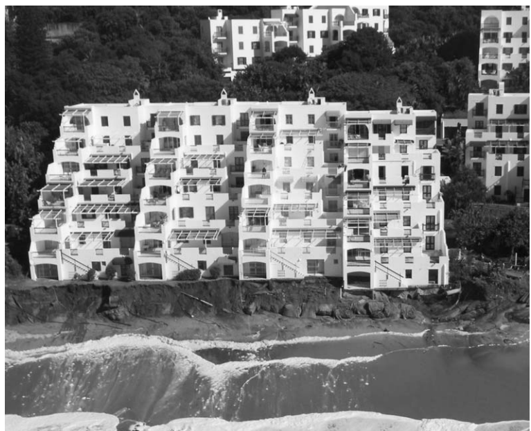
Fig. 3. A multi-storey building in Ballito, which was partially undercut by the storm.
