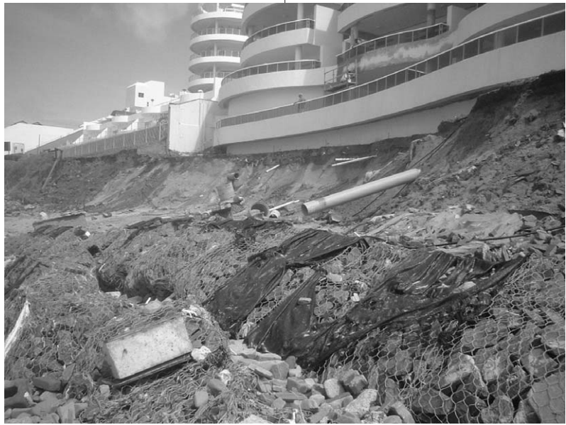
Fig. 2. Beach erosion at Ballito. Note the failed gabions of a previous sea-defence structure. The dune sand on which the structure stands has been undercut, exposing the infrastructure.
